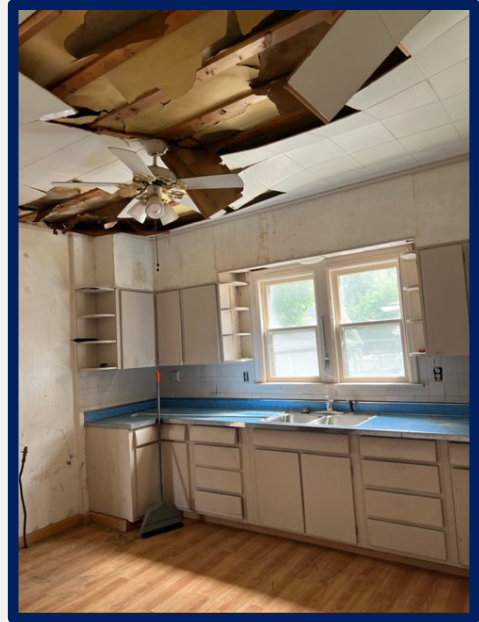
Before Photo: A kitchen set to be remodeled with HOME grant funding.
