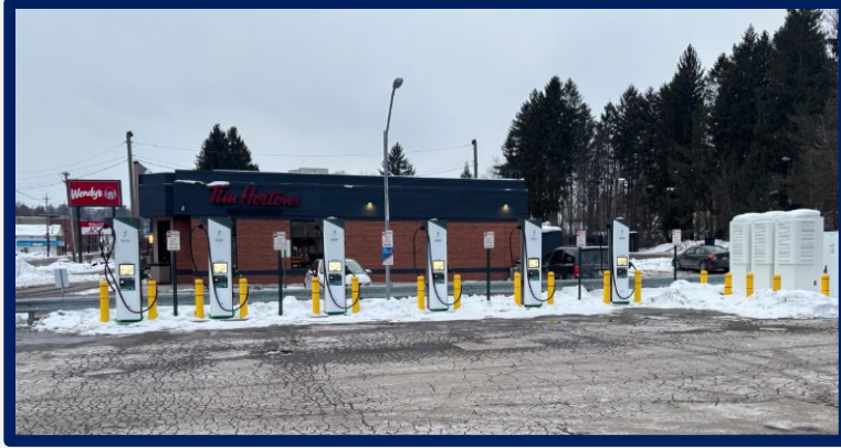
The new EV Chargers now available on East 2 nd Street.
