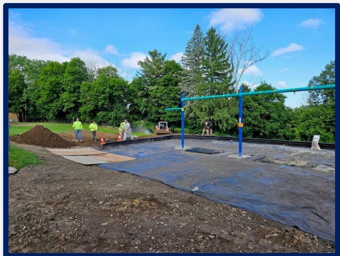
Parks employees installing new playground equipment at the Willard Street Tot-Lot Park.
