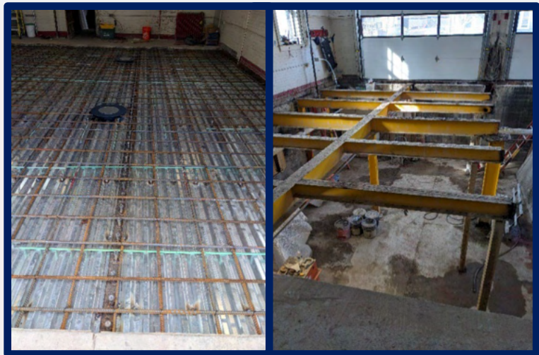
Fire Station 5 on Fairmount Avenue received major updates to its garage flooring in 2024.
