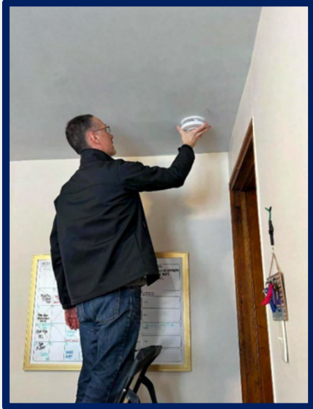
A volunteer installs a smoke detector during the Sound the Alarm Day of Action.
