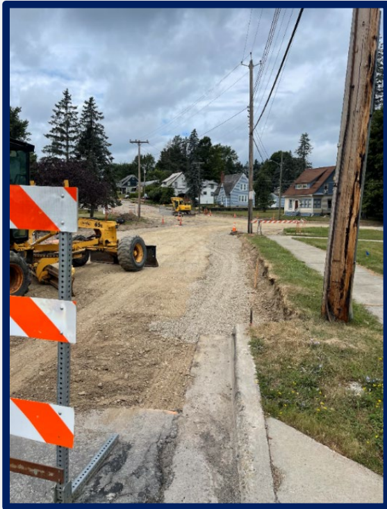
The intersection of Baker & Hazeltine was reconstructed this past summer, enhancing traffic flow and improving safety within the school zone.
